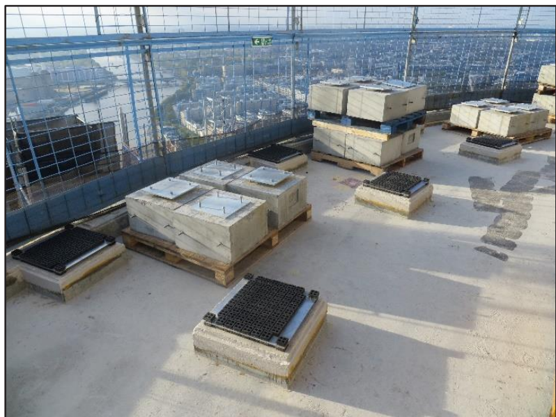
Noise-reducing pads installed on concrete plinths (by others)
